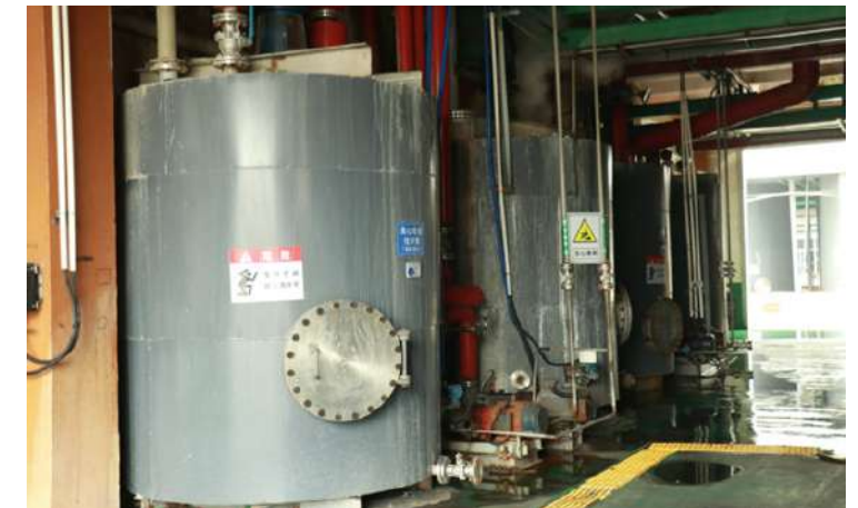
Recycling Technology's water storage equipment
