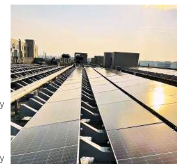
Rooftop distributed photovoltaic systems in factories
